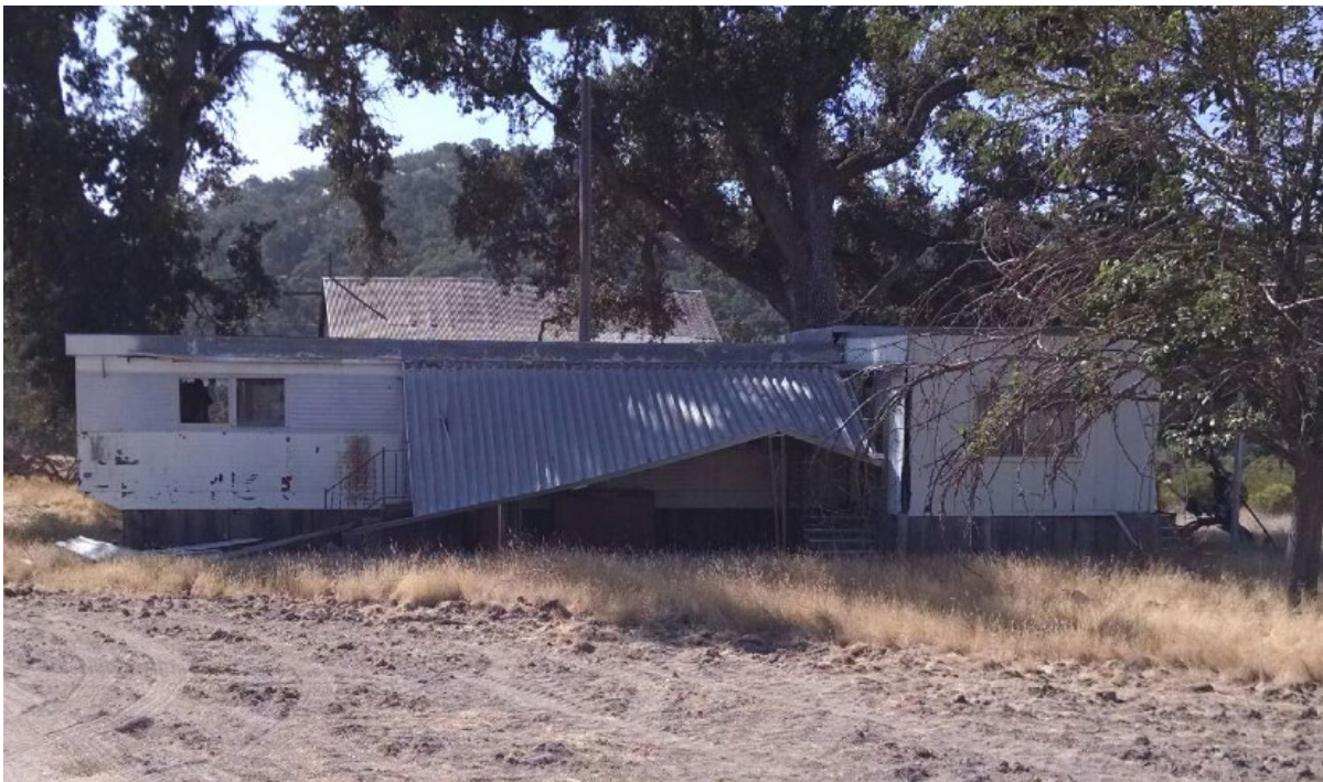
Mobile home with collapsed carport; roof barn in distance, camera facing south (SWCA photo, 9/19/2018).
